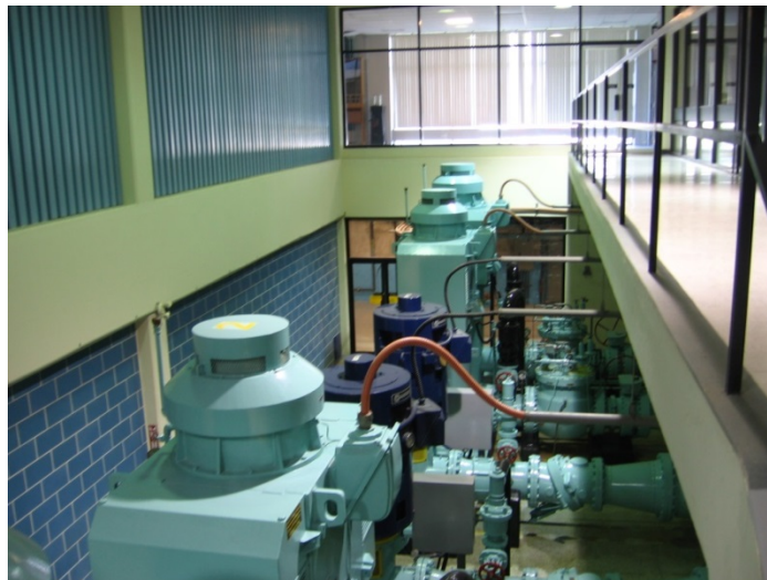
Figure 1: High Lift Pumping Station at WTP
