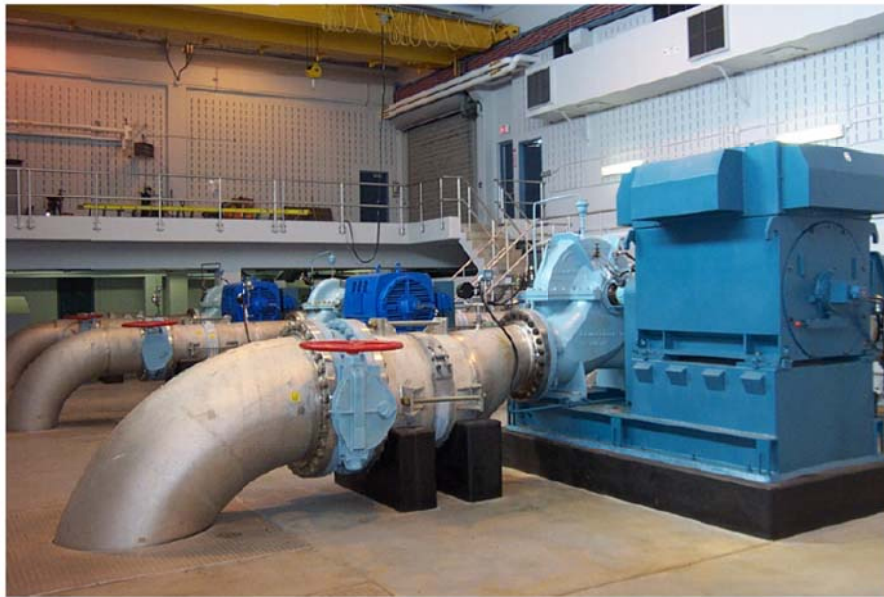
Figure 2: City of London Pumps at EMPS
